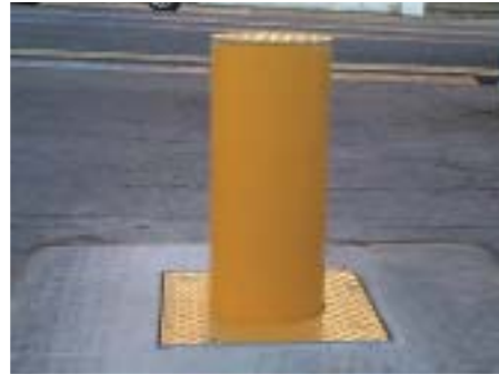
Plain Yellow Hydraulic Bollard securing the exit to a high security public sector building.
