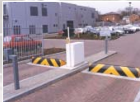
Roadblockers used to secure entry and exit from site.
